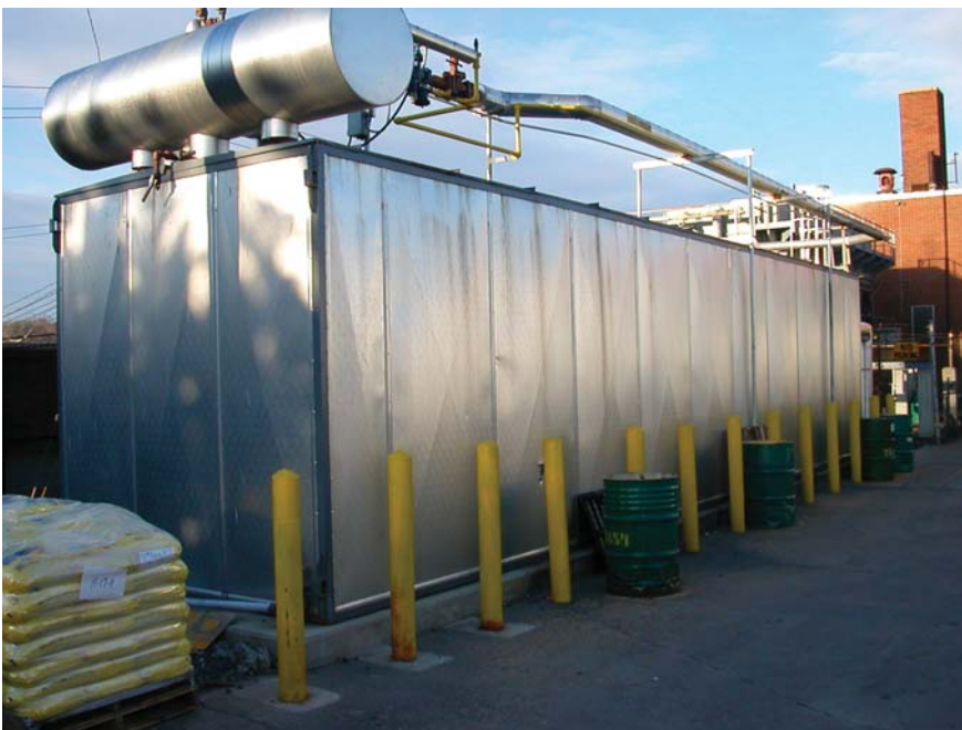
The view above shows a CJ Ice Builder complete with gravity feed ammonia system. This outside installation is located at Cloverland Green Spring Dairy in Baltimore, MD.
