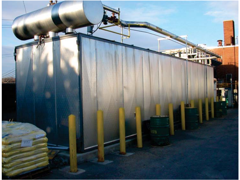
The photo above shows a Chester-Jensen ice builder complete with a gravity feed ammonia system.
